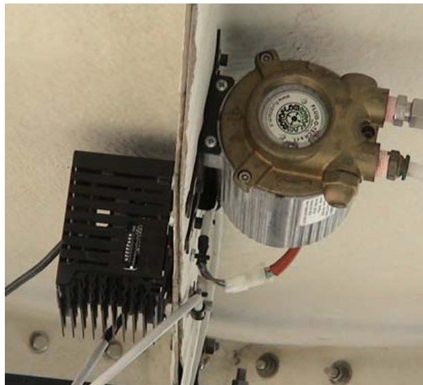
Figure 2.13: Pump and Controller located on underside of the dish.
