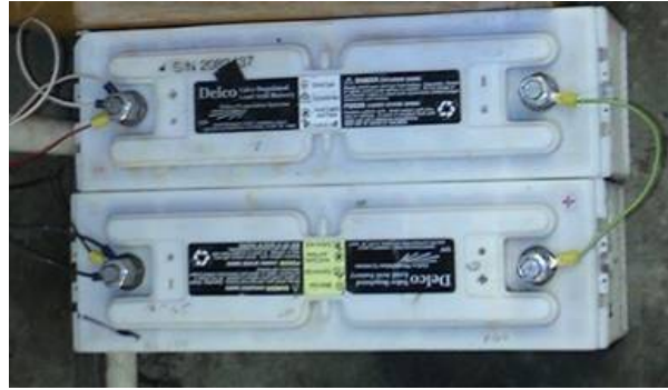
Figure 2.20: Two 12-volt deep cycle batteries wired in series.
