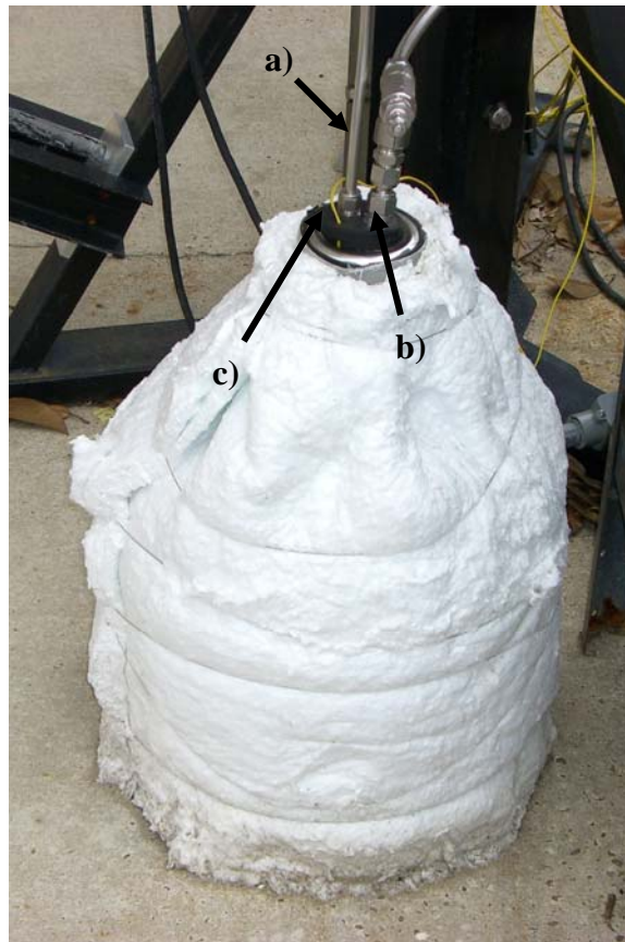
Figure 2.12: Water Tank used for supply water; wrapped in super wool insulation. a) Water line to pump, b) Return inlet from steam turbine, c) Thermocouple insert.
