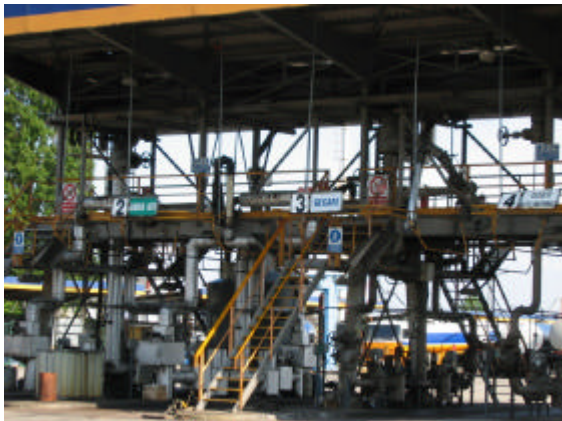
Station de distribution de Gecam
